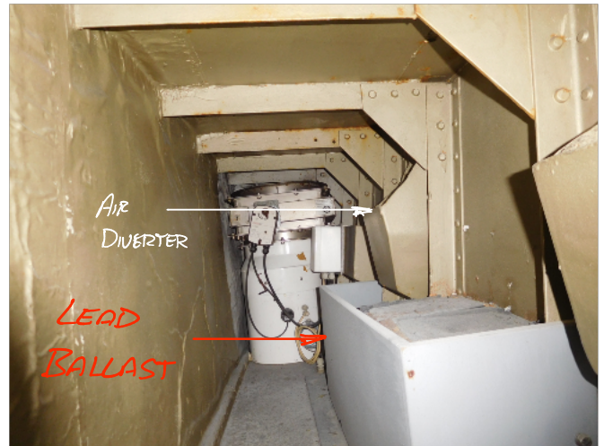
STARBOARD VENT TRUNK
